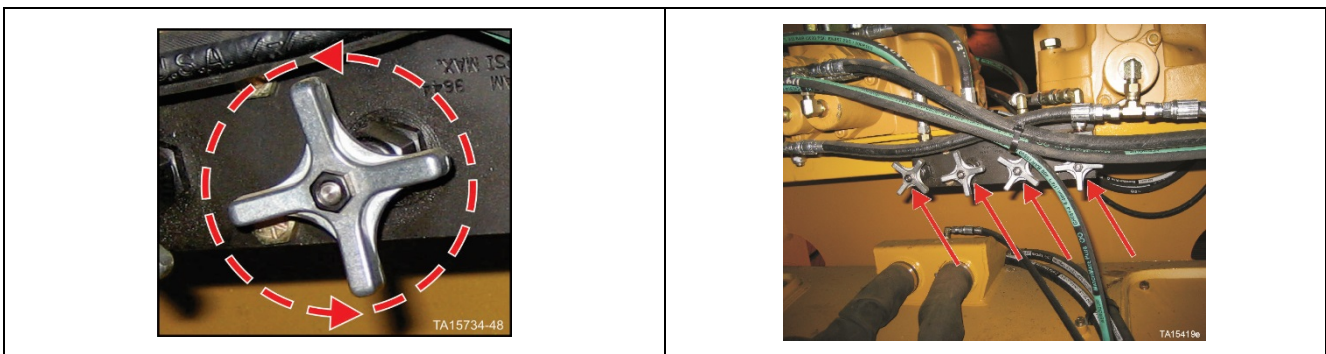
Figure 8. Pressure bleed down valves
