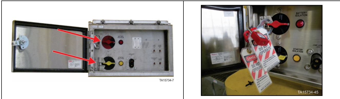
Figure 5. Battery Isolation Box – Battery isolation switch in OFF position with locks in place
